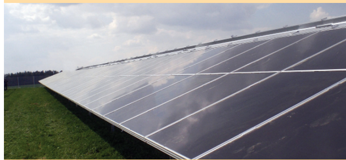
1 MW thin film installation in Munich Germany, April 2009
