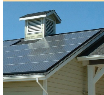
Black frame and low profile racking complement roofline.
